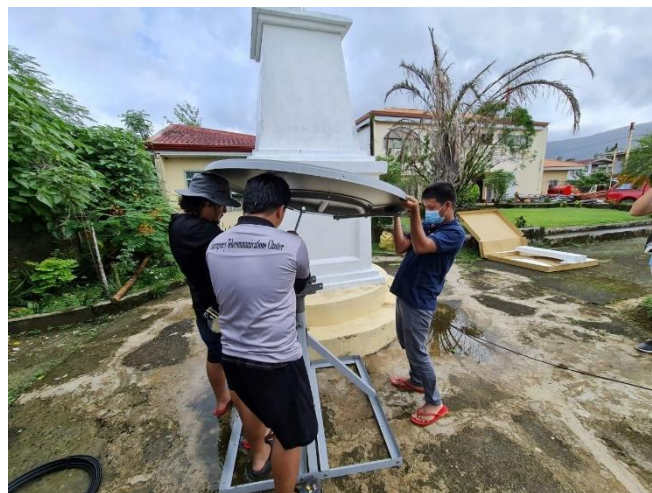
WFP supported the Department of Information and Communication Technology in the installation of Very Small Aperture Terminals (VSATs) in Dinagat Islands. ©WFP/Amirullah Syarif
