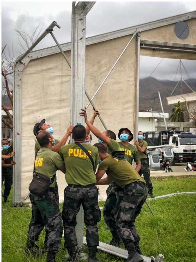
Assembly of mobile storage units at the Provincial Capitol of Catanduanes. Photos courtesy of the Office of the Provincial Capitol of Catanduanes
