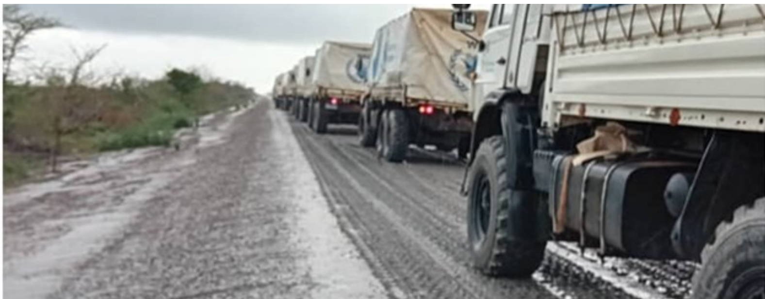
Trucks carrying humanitarian supplies traverse a recently rehabilitated stretch of the Bor-Ayod Road in Jonglei State. This year, WFP has rehabilitated over 260 km of roads across Jonglei, Western Equatoria, Eastern Equatoria, Unity, and Upper Nile States. As of 30 November, WFP had delivered 192,000 mt of food to diverse locations within South Sudan this year, assisting over 4.2 million people. Photo: WFP/ Allan Orimba
